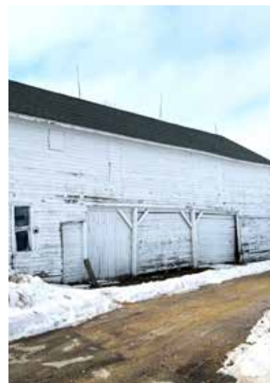
PHOTO (Right) The existing machine shed is nearly falling apart with large gaps in the siding and broken doors and windows.
